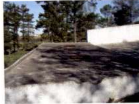
Cistern ( Water Tank )
